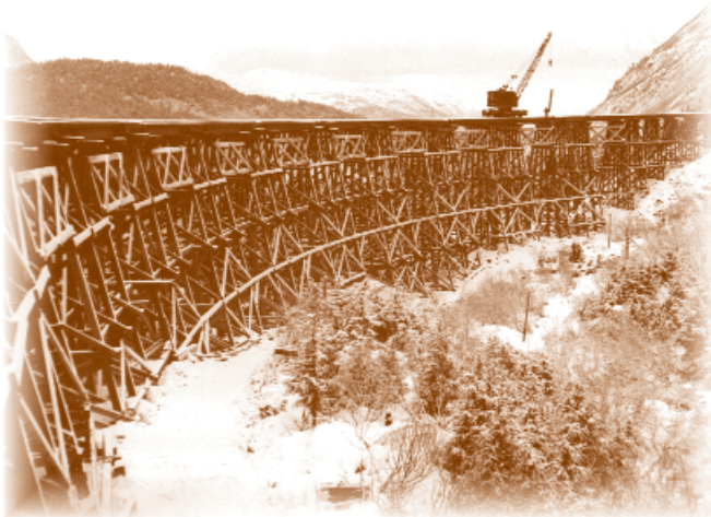
During the winter of 1948, railroad crews conduct brace work to stiffen the Loop District trestle at mile 48.3. in order to ensure continued safe operation. (ARRC photo archive)
