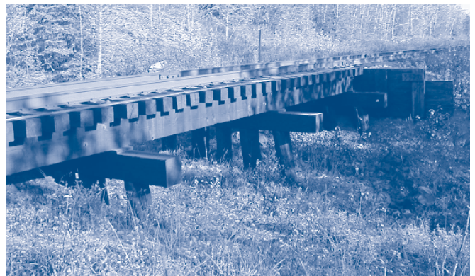
Bridge 337.0 is a 42-foot timber trestle with three 14-foot spans. It crosses a Nenana River drainage eight miles south of Denali Park. Originally built in 1922, it was rebuilt in 1948 and many components have been replaced since then. (2004 ARRC Bridge Survey photos)
