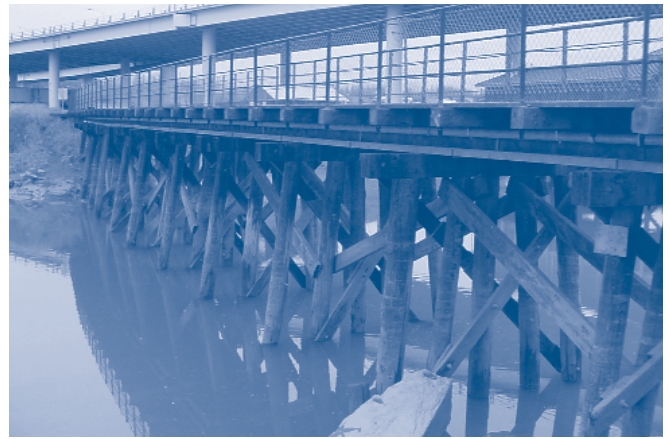
The Ship Creek Pedestrian Bridge at mile 114.6 is in the Anchorage Rail Yard. Originally built in 1916 as a 196-foot bridge comprised of fourteen 14-foot spans, it was rebuilt in 1938 and 1956. Bridge 114.6 was removed from train service in 1987, when it was converted to pedestrian use only.
