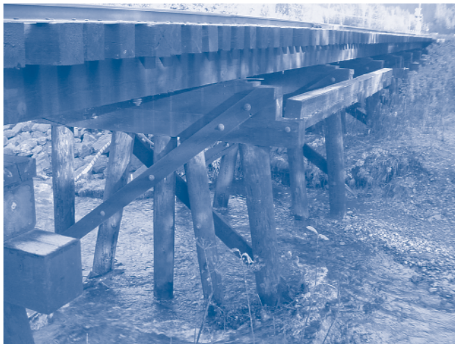
Bridge 6.60 is a 135-foot timber trestle with nine 15-foot spans. It crosses Bear Creek near Seward. Originally built in 1917, Bridge 6.6 was rebuilt in 1953, and most components were replaced in 1985.
