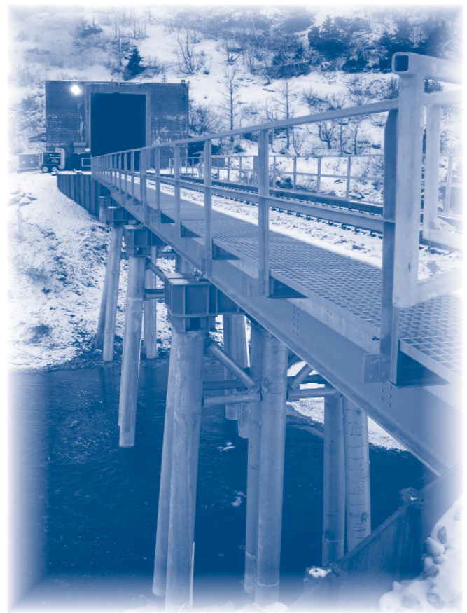
A steel bridge replaced the timber bridge at mile F5.7 in late 2006.
