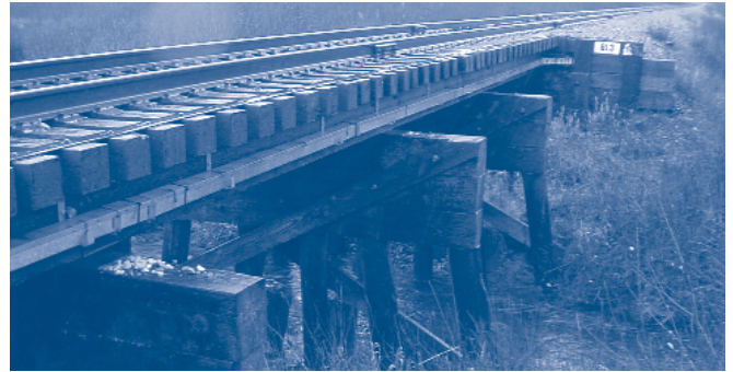
Bridge 61.3 is a 54-foot timber trestle comprised of two 15-foot, one 14-foot and one 10-foot spans. It crosses a Placer River tributary near Portage. Originally constructed in 1919, it was rebuilt in 1950, and many components have been replaced since then.
