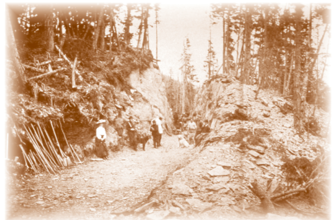
Alaska Central Railroad construction gets underway in 1904 near Seward. (ARRC photo archive)
