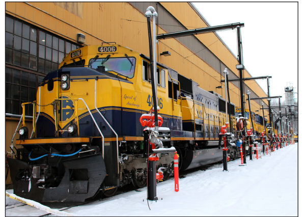
Fueling stations installed along the Diesel Shop.
