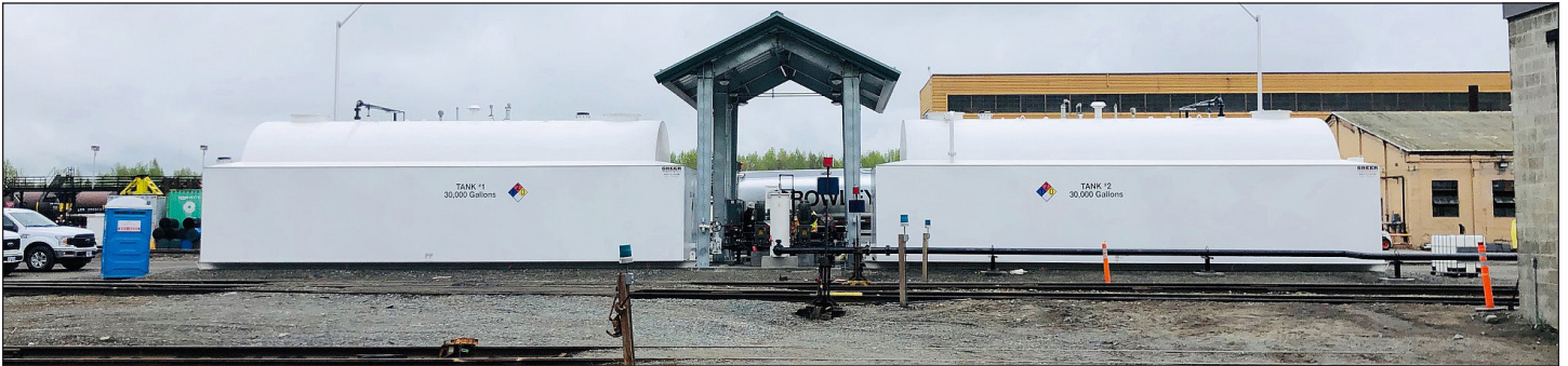
Storage tanks placed in January 2020 are hooked up to a pump house and above-ground piping.
